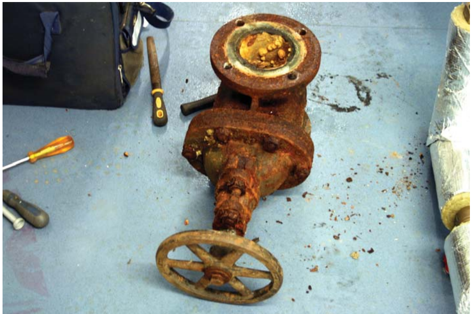
Figure 3. Image of a corroded valve removed from a water system. Image courtesy of Pete, from Liverpool, UK. This file is licensed under the Creative Commons Attribution 2.0 Generic license.
